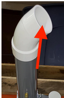
Figure 15) Protecting Fan Outlet From Animals
